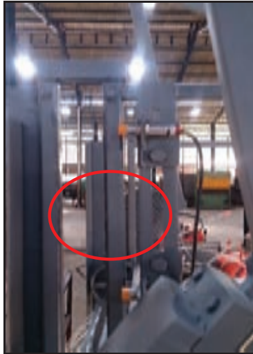
Figure 12 Proximity sensor's set up at the moving path of the DC motor.
